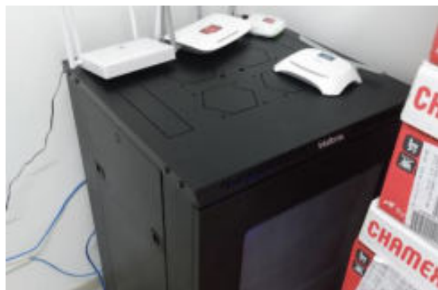
Figura 3 Links internet GSTN, CSI e Rack com Mikrotik instalado
